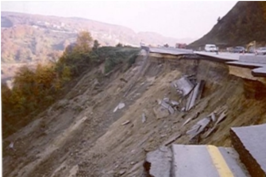
Figure 14. Landslide on E5 Highway in Duzce Earthquake
