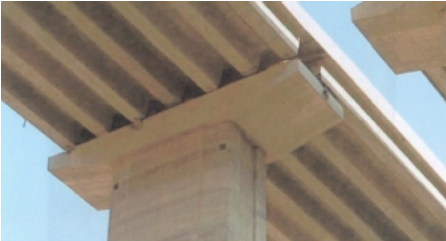
Figure 26. Movement between the piers and the girders of Bolu 1 Viaduct
