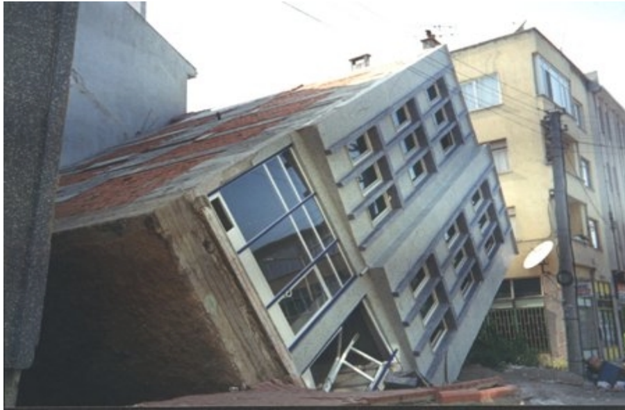
Figure 12. Overtumed buiding in Adapazari due to weakened/liquefied foundation
