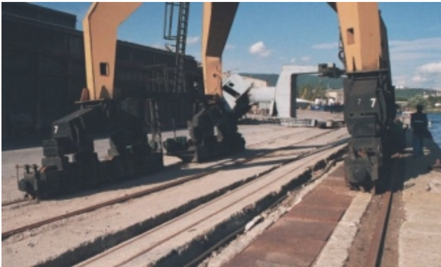
Figure 30. Damage at Derince Port in Kocaeli Earthquake
