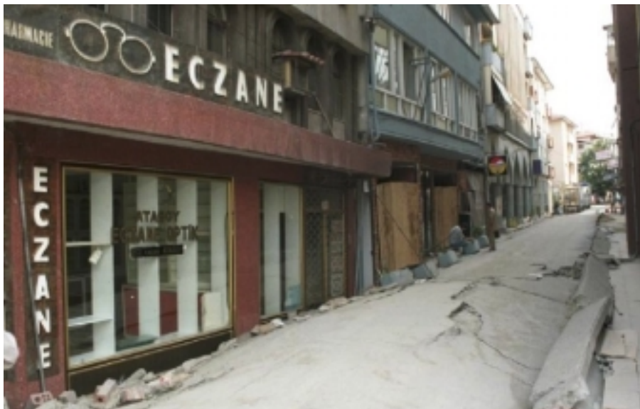
Figure 13. Building in Adapazari that sank into the ground and the displaced soil heaved
