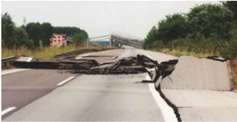
Figure 23. Damage to road surface on TEM Highway in Kocaeli Earthquake
